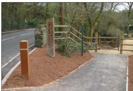
▲ Improving the entrances to the nature reserve and making access safer was a key priority
